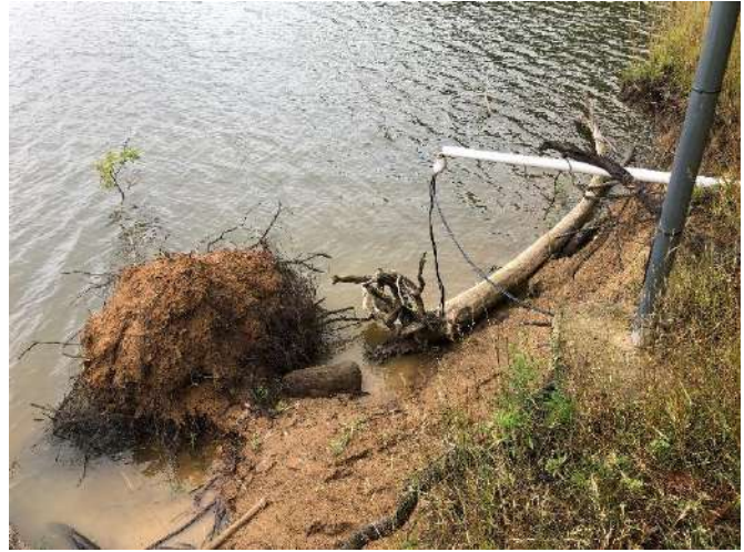
Excessive erosion along Hoover Reservoir's shoreline.
