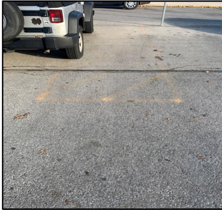
FIGURE 5. ACCESS AISLE NOT MARKED TO DISCOURAGE PARKING (WOODWARD PARK, LOT 3)
