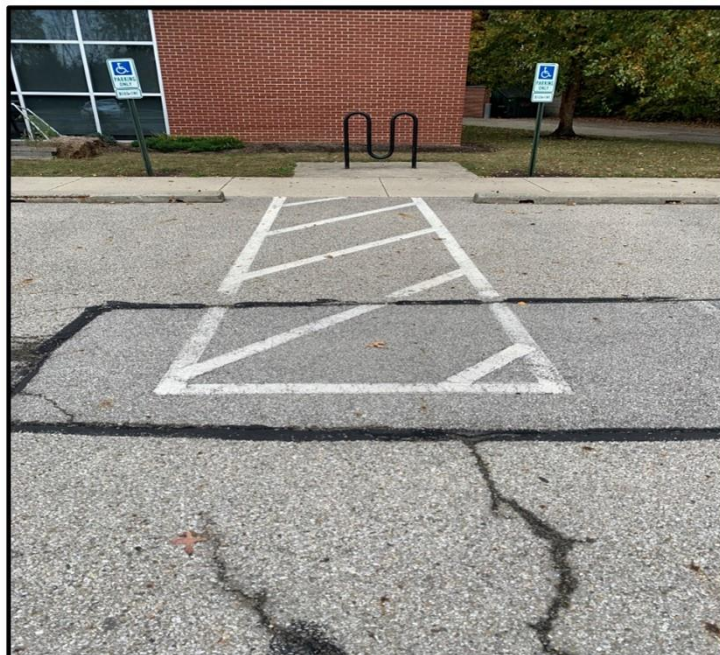
FIGURE 6. VERTICAL DISCONTINUITIES IN ACCESS AISLE (LAZELLE WOODS PARK, LOT 2)
