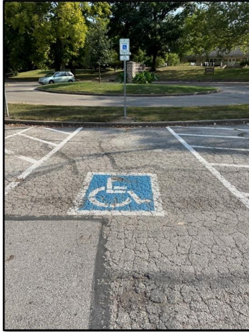
FIGURE 3. VERTICAL DISCONTINUITY (WHETSTONE PARK, LOT 2, SPACE 3)
